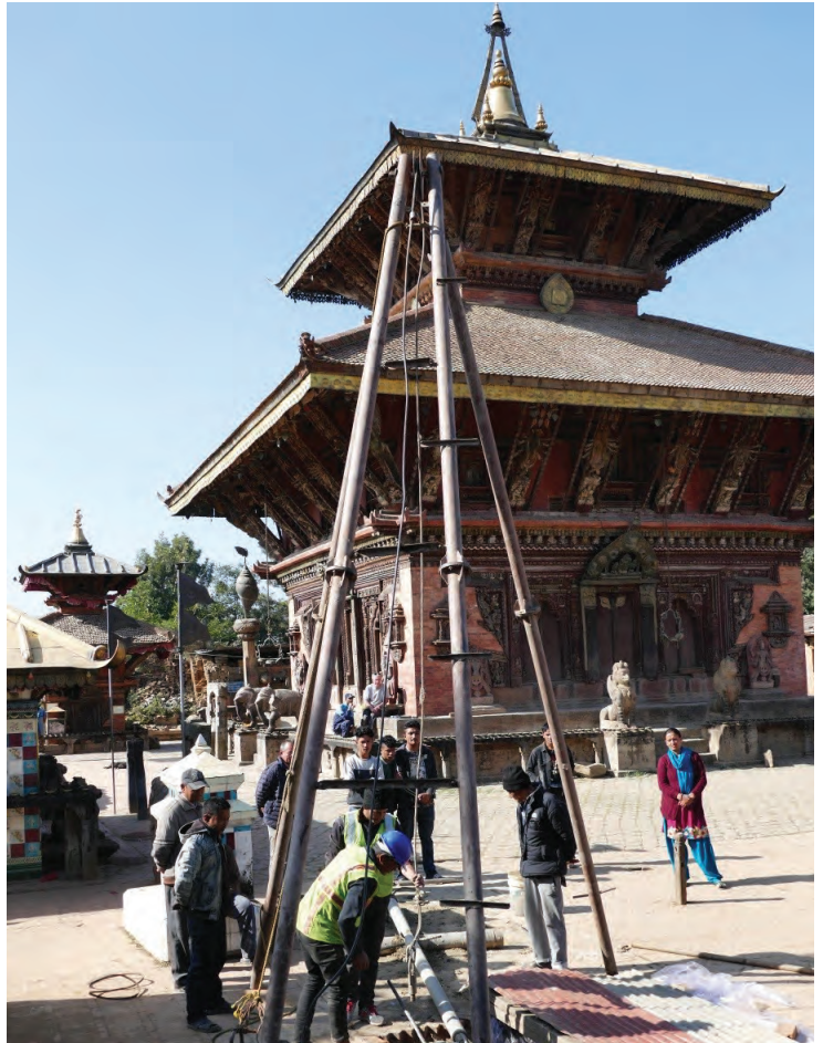
Geotechnical sampling next to the Changu Narayan Temple in Kathmandu’s World Heritage Site. PHOTO: DURHAM UNESCO CHAIR.
