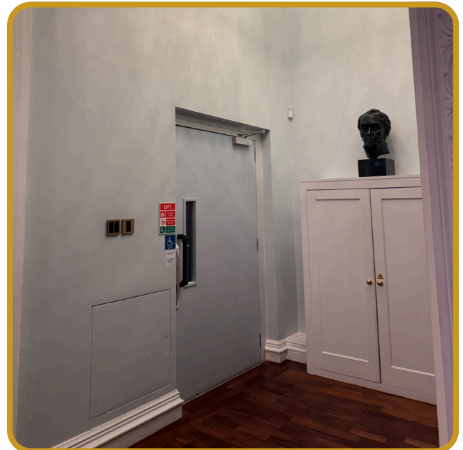
Platform Lift - No. 11 Lobby
