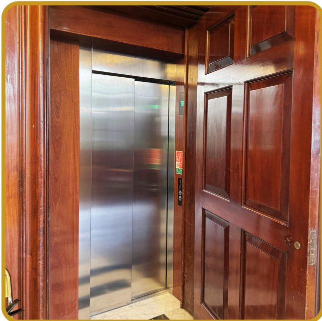
Passenger Lift - waiting area
