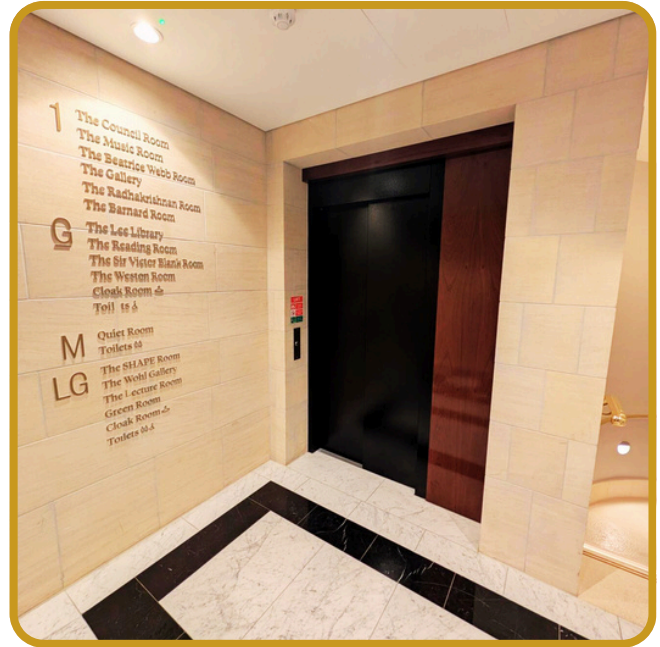
Platform Lift - No. 10 Lobby
